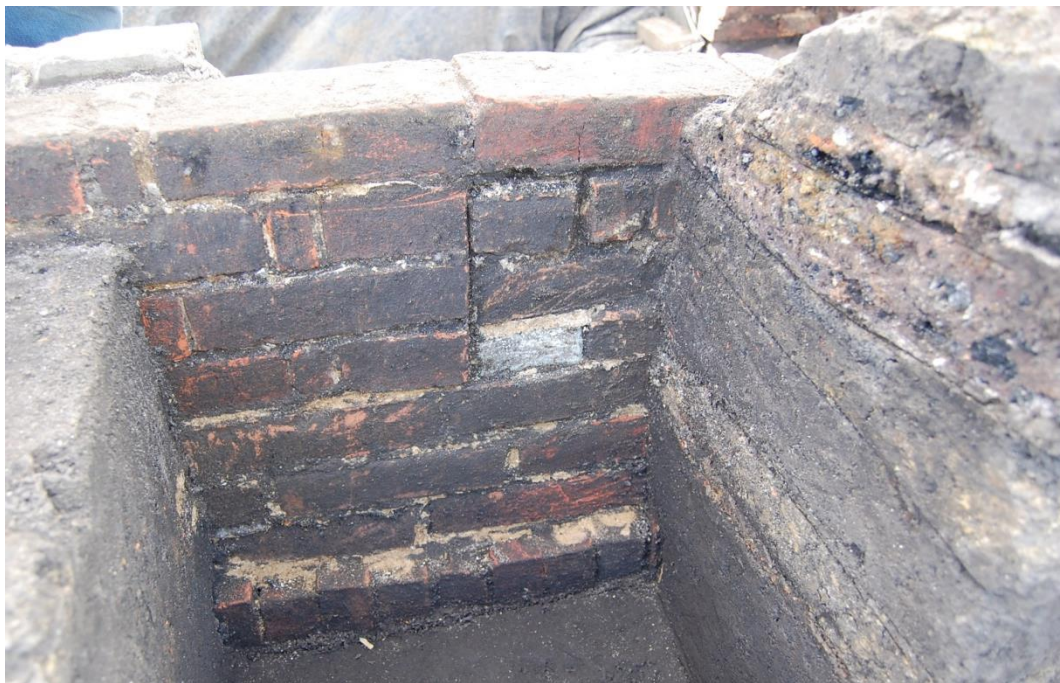
Figure 34. Details of the exterior face of the east foundation wall of House B (within Test 10) showing the south edge an apparent infilled opening—indicated by the butt joint. While this opening may represent the location of a door sill that later was relocated, its position does not correlate well with the suspected floor level on the interior of the house. Also of note is the partial spread footing, which only found on this side of the house foundations.
