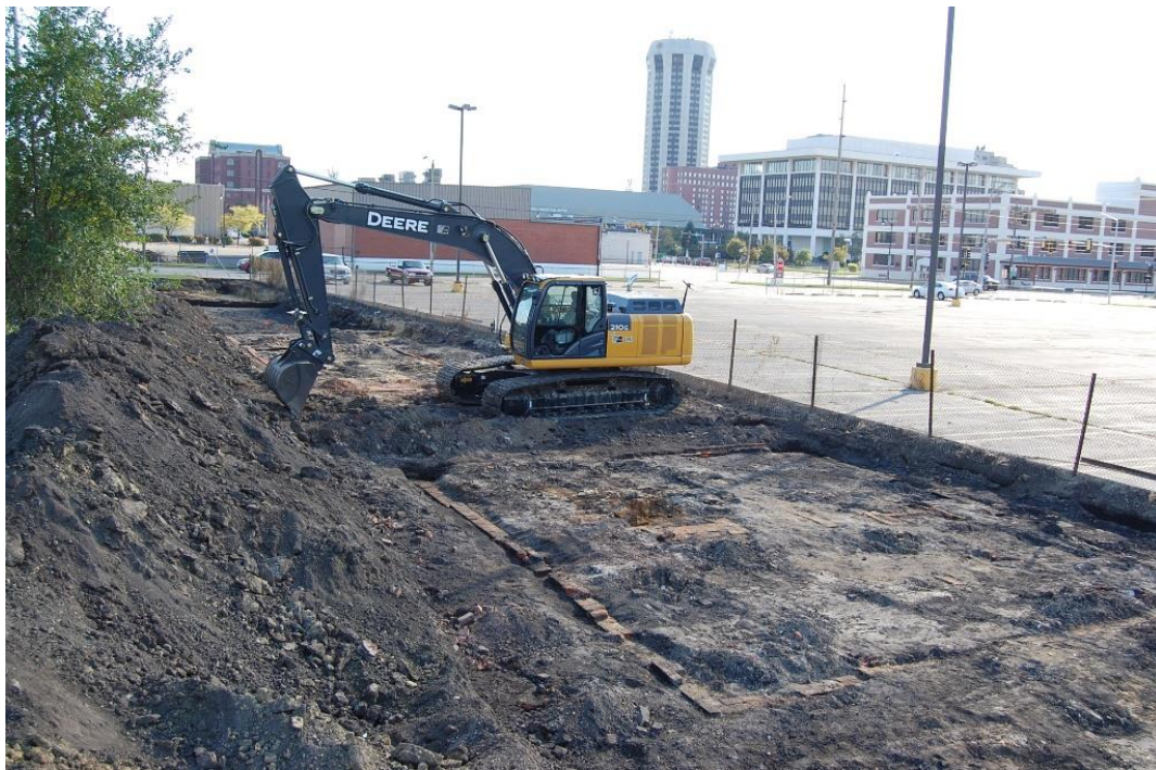
Figure 9. Phase II archaeological investigations in process. Top: Initial investigations opening area north of House A, using a small tractor-mounted backhoe. Bottom: Continuation of stripping near House D, using a larger track hoe. The foundations of Houses A, B, and C are located on the side of the track hoe. Springfield's central business district appears in the background of this view.
