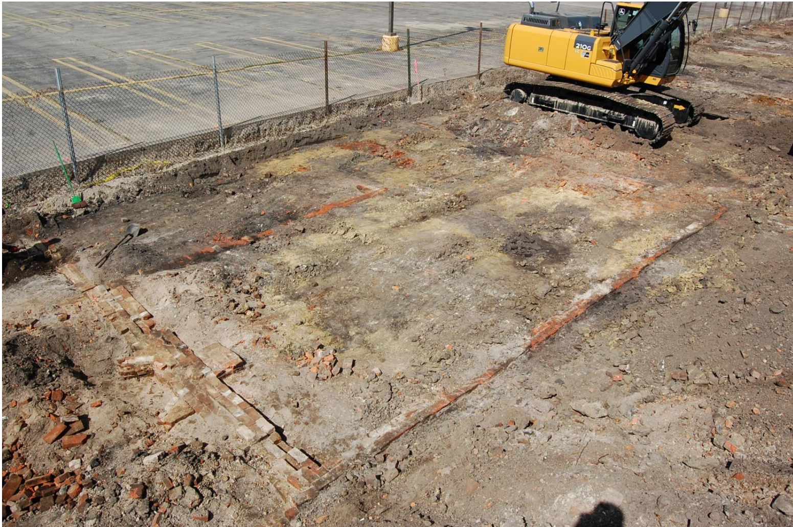
Figure 14. View of House C during initial Phase II exploratory investigations (looking northwest, fall 2014). The upper part of the brick perimeter foundations of the original house (Feature 1) has been exposed. The south end of House C directly abutted House B, whose foundation remains can be seen at lower left.
