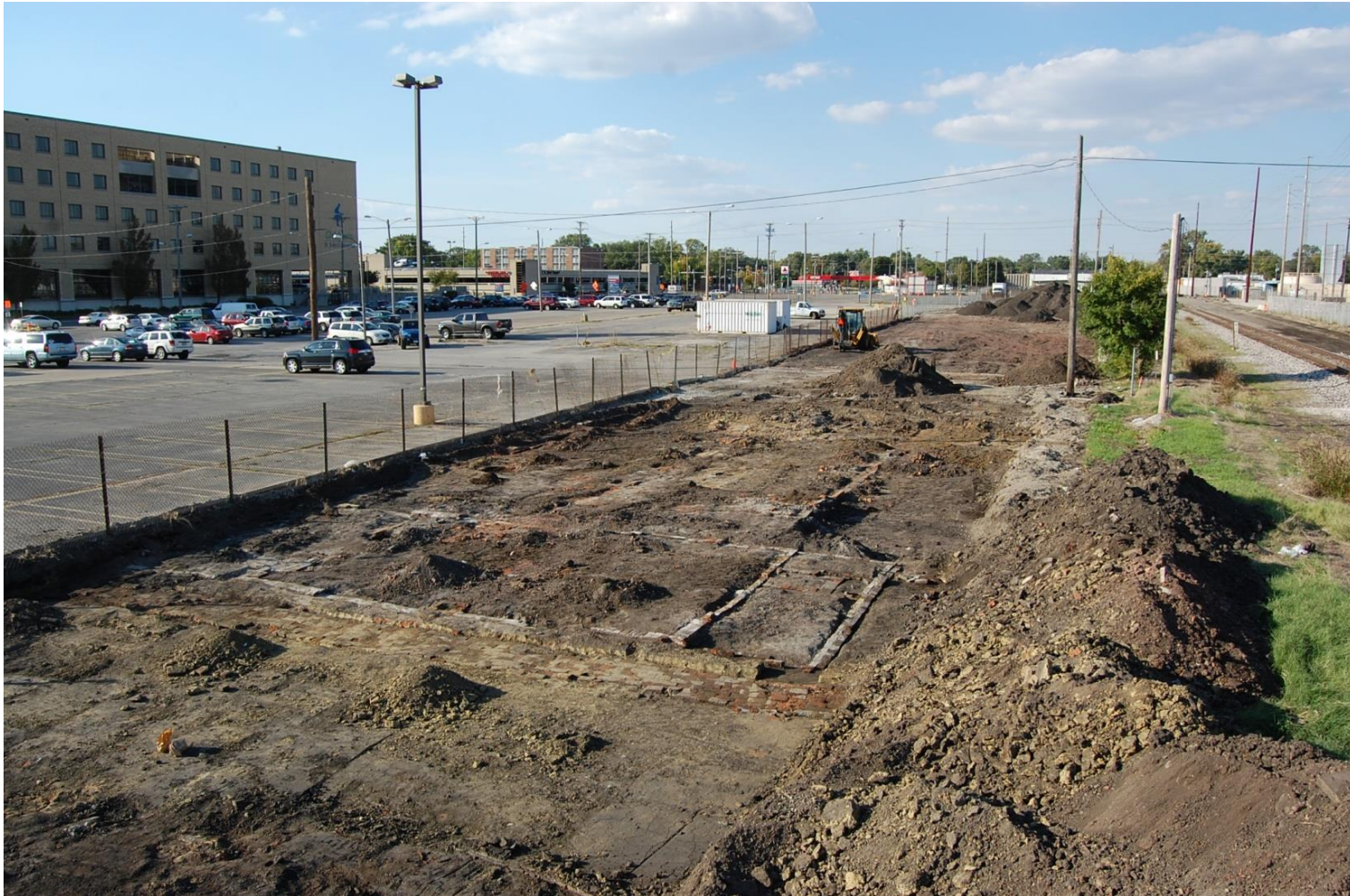
Figure 10. View of Site 11SG1432, looking north, after being stripped of overburden for the 2014 Phase II testing. House E appears at lower center of this view, while Houses F and G are located north of it. The small dirt pile rests on the edge of the abandoned stretch of Mason Street, with the backhoe in the background across the street. The backhoe is sitting on Site 11SG1433.
