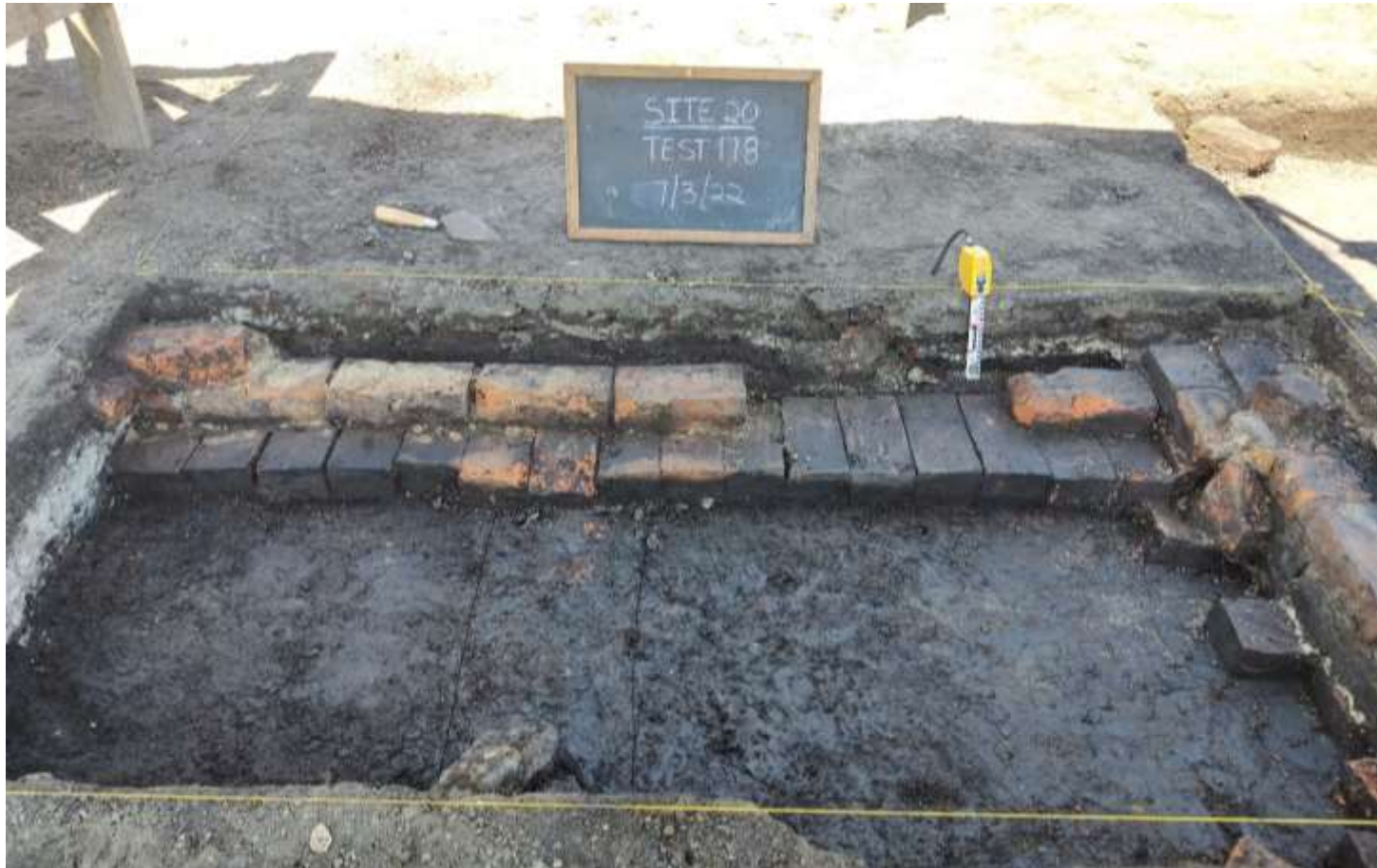
Figure 321. Northwest corner of house, the Sappington illustrating method of construction used for the brick perimeter foundations (Feature 47). The foundations had a base course of header brick, which served as a nominal spread footing. The main foundation wall was only one wythe thick.
